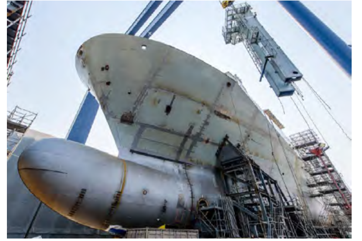
Bottom view of the hull of the future HMCS Protecteur, the longest ship ever built in Canada.
